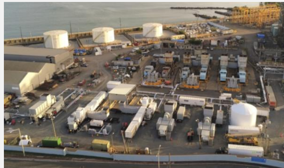
Palo Seco temp power
